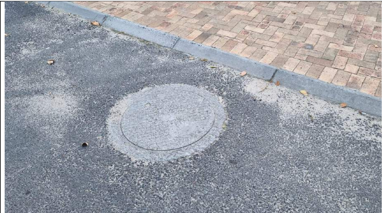
Figure 8.3 B- Manhole on existing pipeline along Kolgans – upgrade required.
