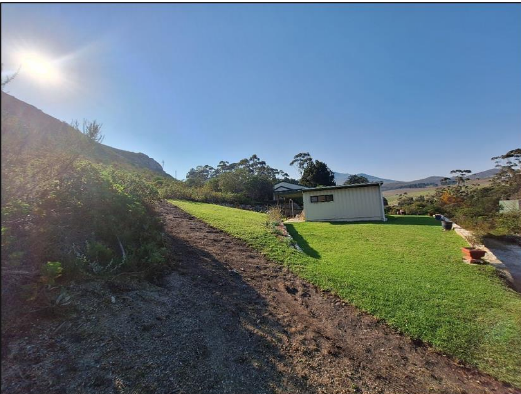
Photo 5: Site 2 – indigenous vegetation cleared and area terraced to develop a single residential dwelling
