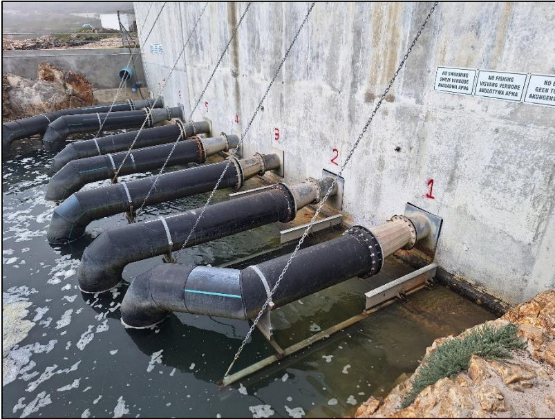
Figure 3a. Photo showing existing pumphouse and seawater abstraction lines
