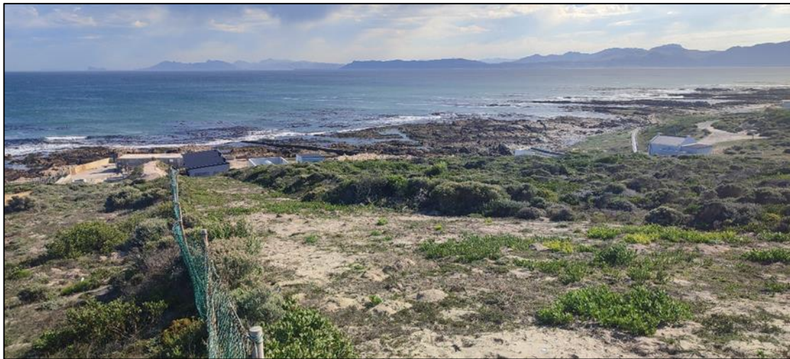
Photo 5: View west along proposed pipeline route to existing pumpstation, with brushcut area to the right (north) of the fence (Helme, 2024).
