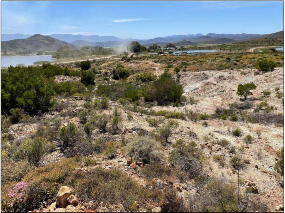
Photo 1: View of the upper northern section characterized by degraded land with a high susceptibility to erosion.
