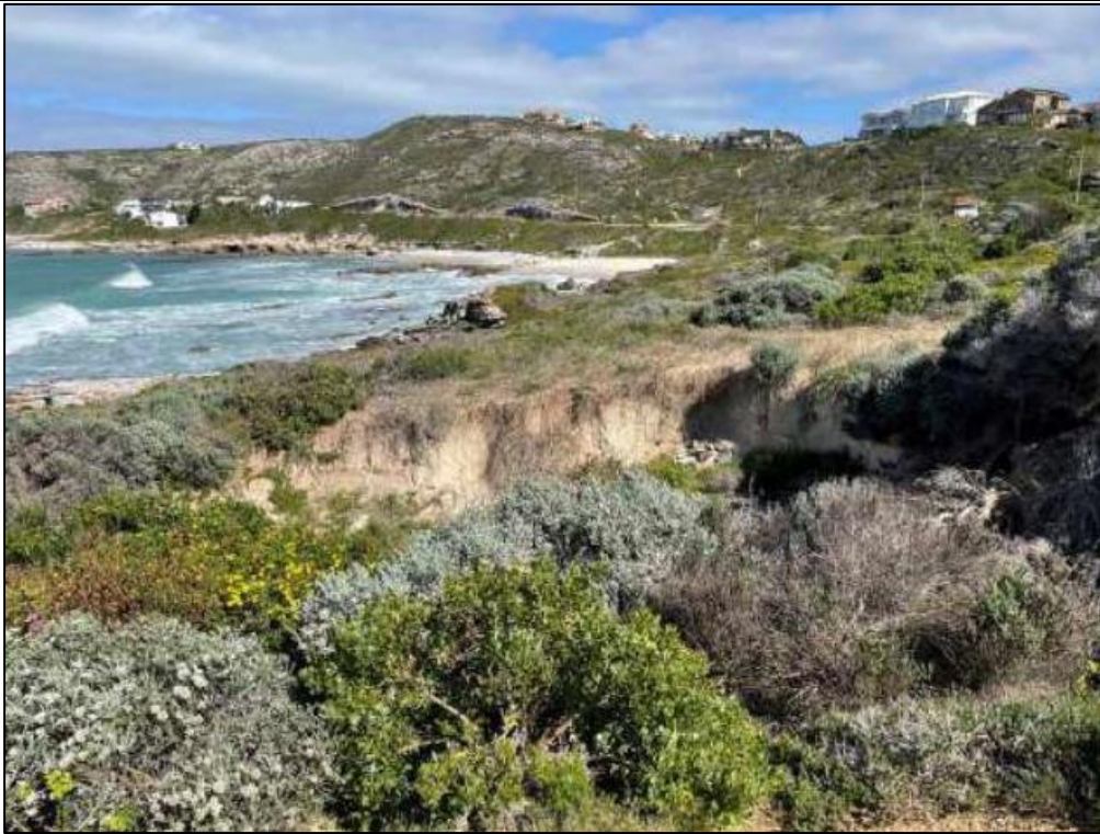
Figure 34: Deep erosion ditch in the foreground created by the stormwater outlet on site.
