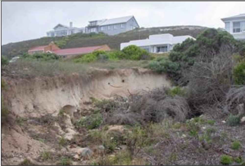
Photo 2. This image shows erosion of the accumulated aeolian sand. Note the thickness (depth) of the sand. The cause of the erosion is the egress of stormwater from a culvert at the edge of Marine Drive. ( source : McDonald, 2023)
