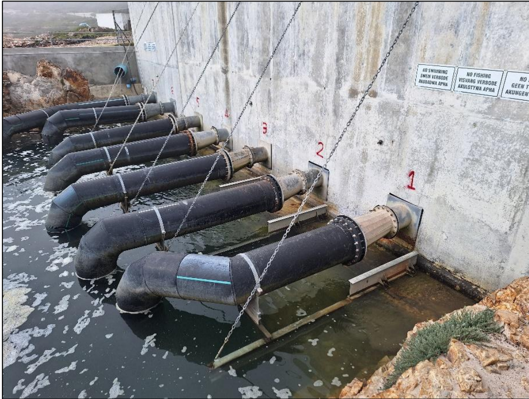
Figure 3-1. Photo showing existing pumphouse and seawater abstraction lines.
