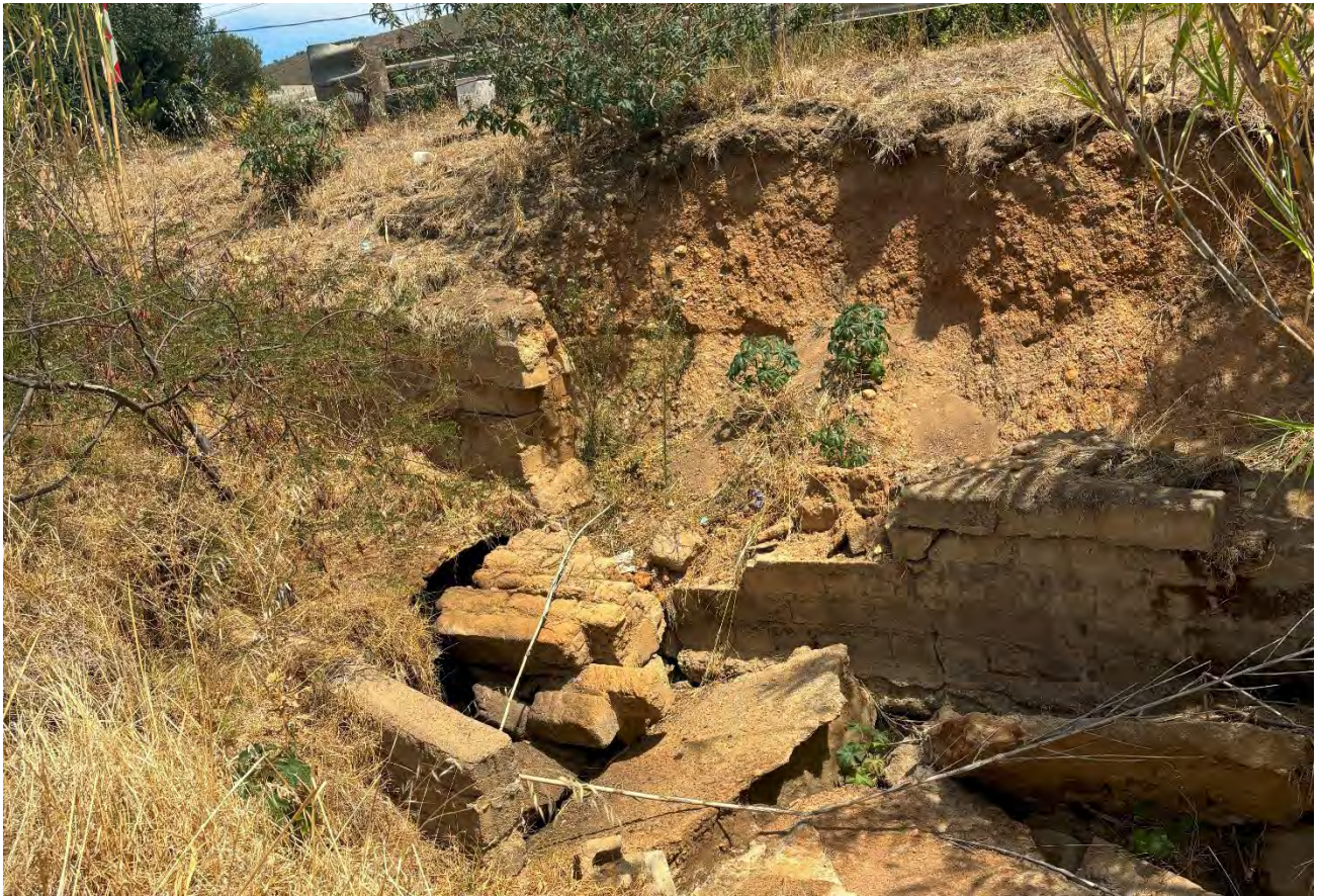
Figure 5-17: Point at which the Krom River enters the proposed development site by means of a degraded stormwater channel. Bank stabilisation measures have collapsed and are currently blocking the stormwater pipeline.
