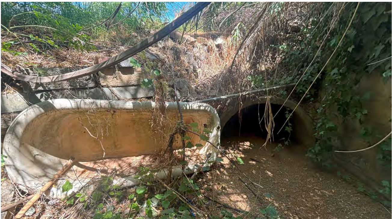
Figure 5-18: Point at which the Krom River emerges from the underground pipeline in the northern portion of the site. Rubble has been used for infill and bank stabilisation.
