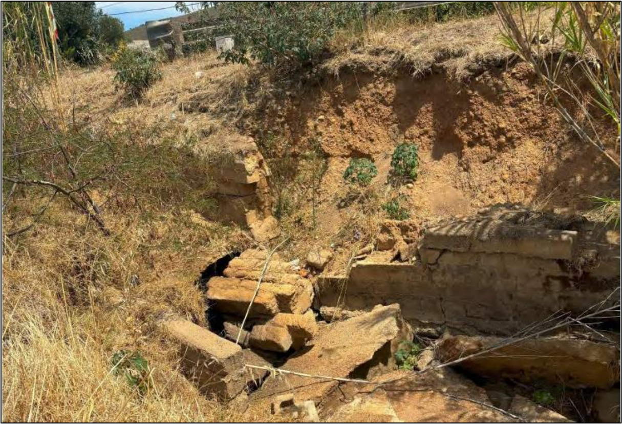
Figure 21: Point at which the Krom River enters the proposed development site by means of a degraded stormwater channel. Bank stabilisation measures have collapsed and are currently blocking the stormwater pipeline. Source; (Van Zyl and Brunings, 2025).
