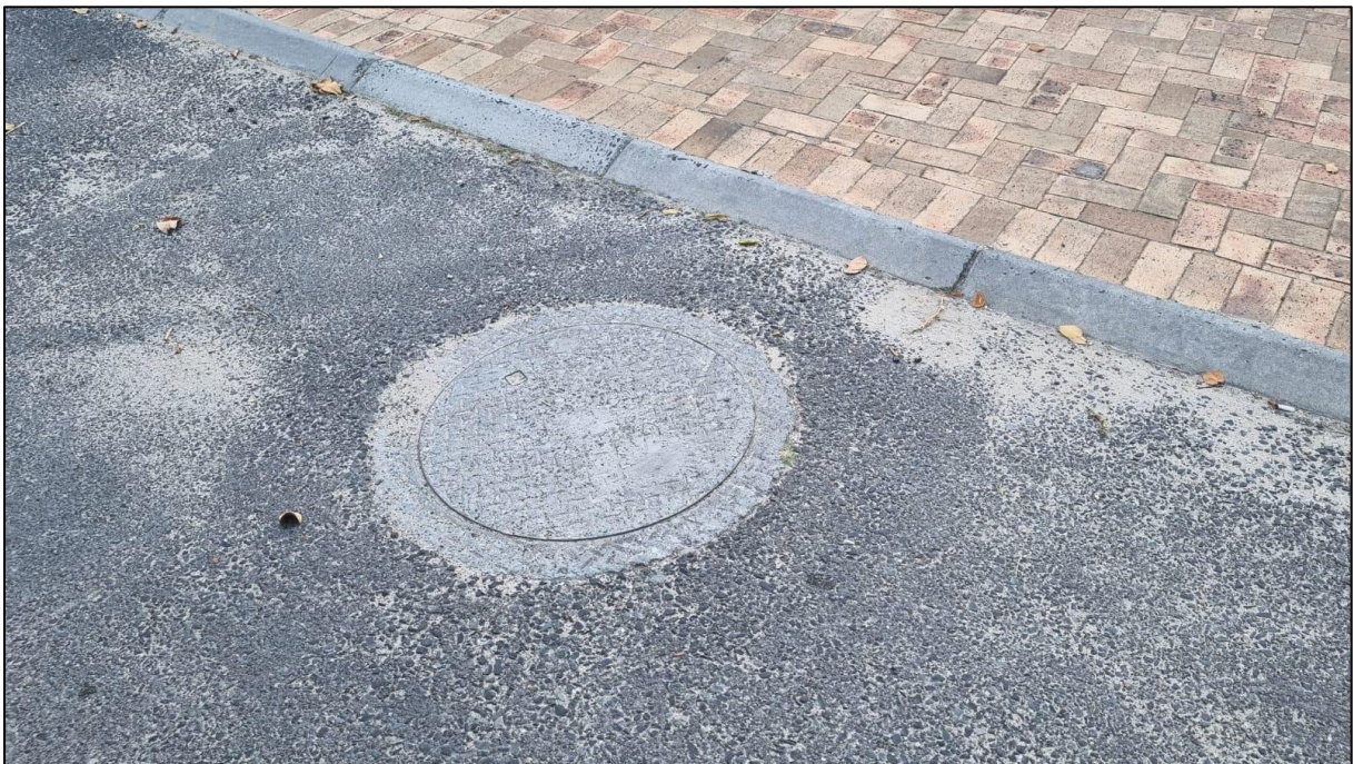
Figure 7.3-B - Manhole on existing pipeline along Kolgans – upgrade required.
