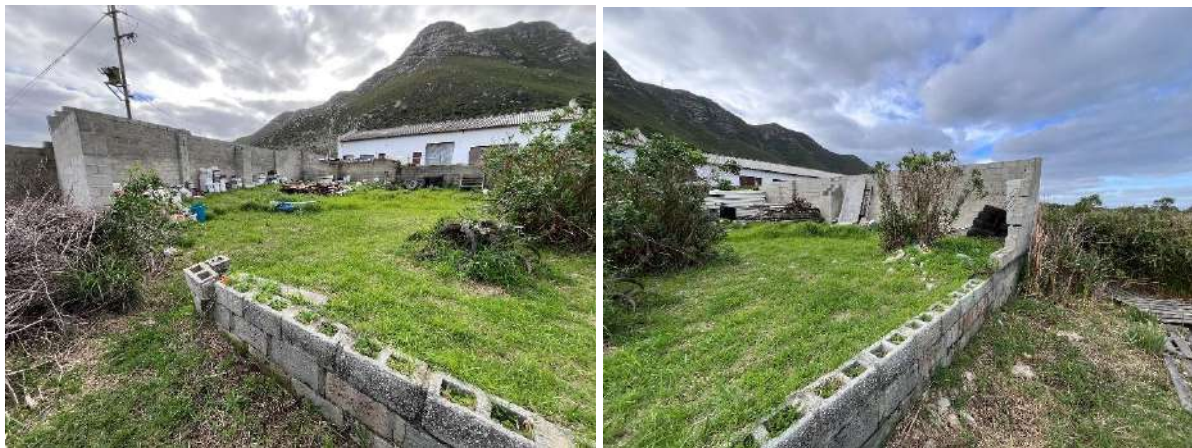
Figure 3.18: A derelict building associated with the main dwelling that was built within the wetland.
